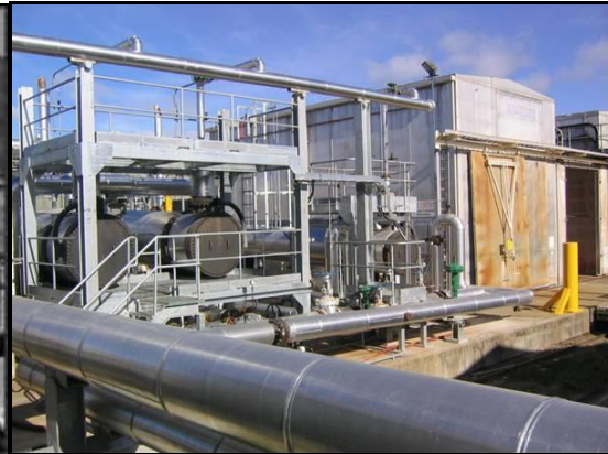
Figure 20: A geothermally heated timber drying kiln
